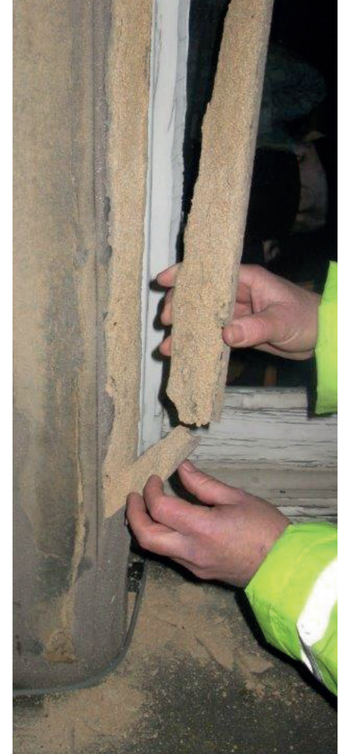
Damaged stone window architrave
